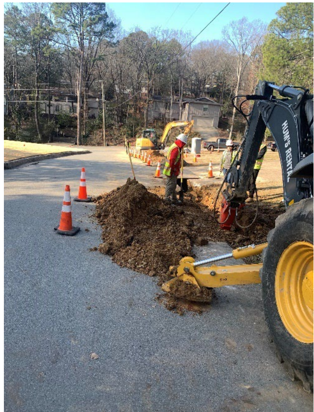
In some locations, the new pipe is installed along or within the edge of the asphalt street pavement.
