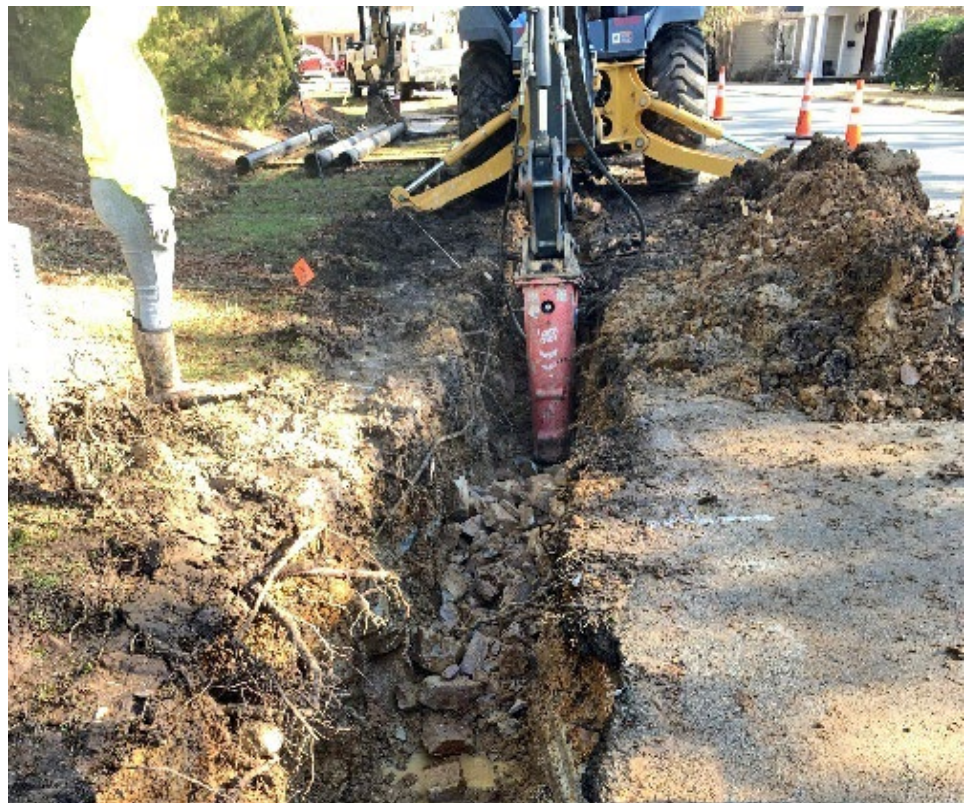
A rock breaker was required in areas to help excavate the pipe trenches.
