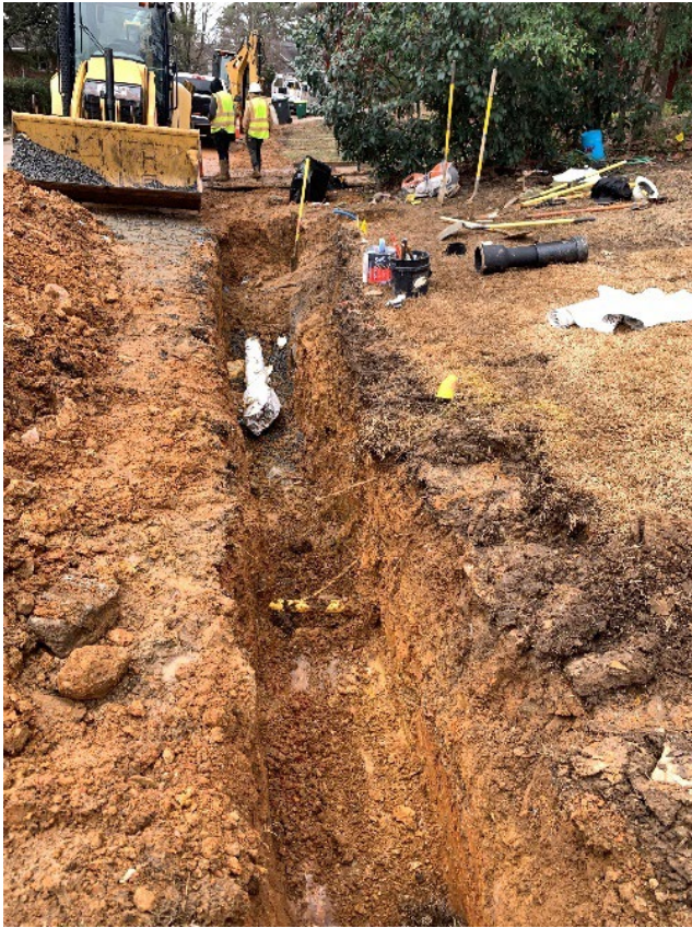
Trenching for new 6-inch main. The contractor trenches well ahead of where pipe is to be installed to check for existing obstructions/conflicts and to allow room for maneuvering/adjusting the new pipe where necessary. Note the gas main (colored yellow) that was exposed.
