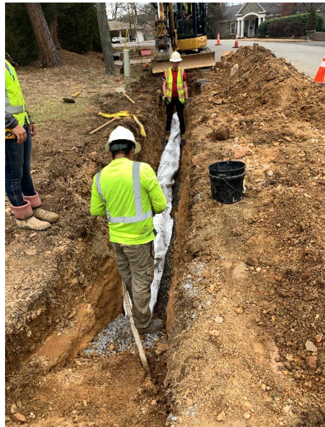
New 6-inch main placed in trench with poly-wrap. The poly-wrap is being inspected and the joints taped.
