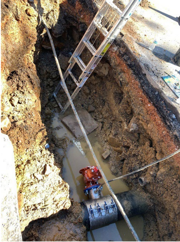
A 6-inch tap being prepared on an existing 12-inch main. The tapping sleeve is being pressure tested prior to the actual tap being made.
